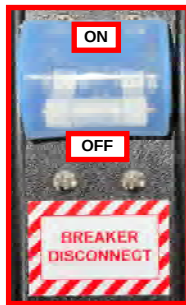
Circuit Breaker Main ON/OFF
