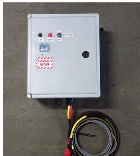
DC Control Box
